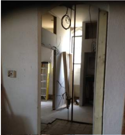
View the other way in the narthex to where the old vestry/storage room was. This is the outline of the loo going in – you can see into the disabled loo area.
